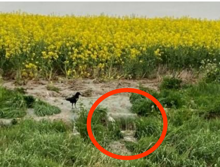
Sewage flowing from burst rising main between Haslingfield and Haslingfield Sewage Works in 2022
