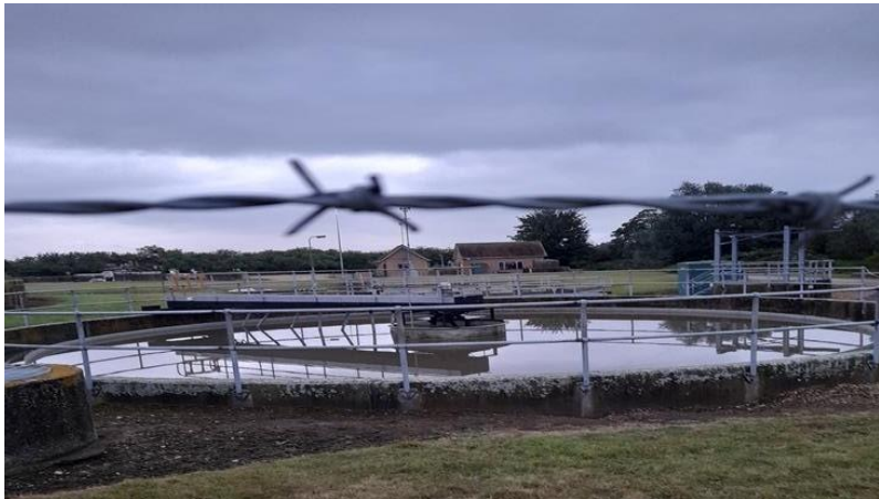
Overflow tanks at Haslingfield Sewage Works full to the brim
