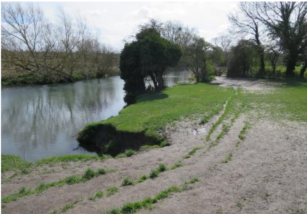
21. An example of erosion to the riverbank and riverside path.
